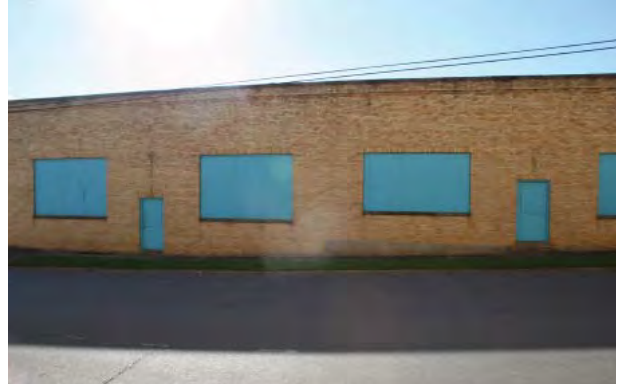
Figure 2-112. A boarded-up commercial building on Jones Street, west of the high school. Source: John Milner Associates, Inc., 2007.
