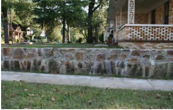
Figure 2-111. A retaining wall on the corner of S. Park and W. Sixteenth Streets. Source: John Milner Associates, Inc., 2007.
