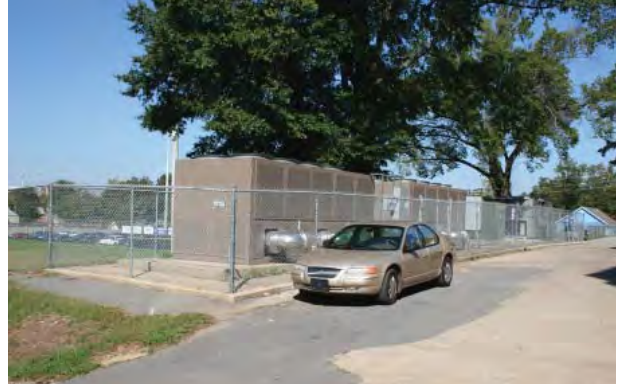
Figure 2-131. Pavement in drives is cracked and patched. Source: John Milner Associates, Inc., 2007.
