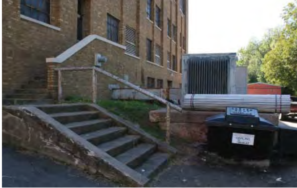
Figure 2-130. Damaged stair cheekwalls. Source: John Milner Associates, Inc., 2007.
