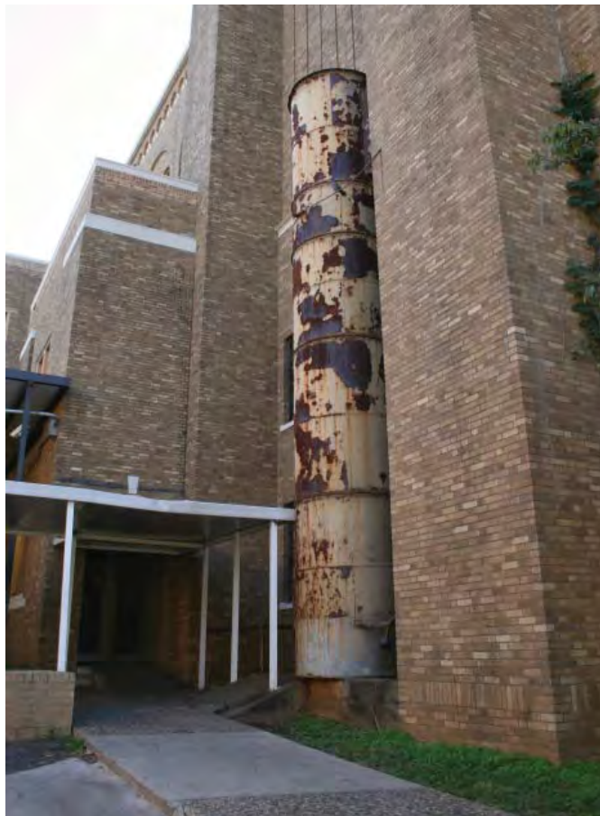
Figure 2-86. One of the features found at the back of the building is this spiral fire escape slide enclosed in metal sheeting, presumably original to the building. Its twin is located on the opposite corner on the same side of the building. Source: John Milner Associates, Inc., 2007.
