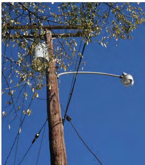
Figure 2-166. Street lighting attached to a utility pole. Source: John Milner Associates, Inc., 2007.
