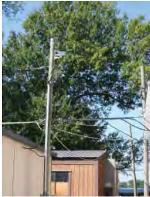
Figure 2-143. Utility poles between the modular structures on the southwest side of the school. Source: John Milner Associates, Inc., 2007.
