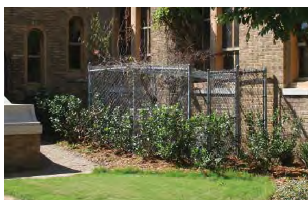
Figure 2-62. Chain link fencing and shrubs secure and partially conceal HVAC equipment near the front entrance of the school. Source: John Milner Associates, Inc., 2007.
