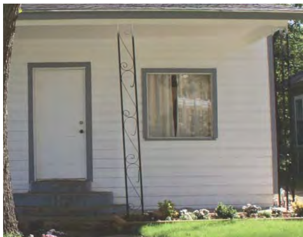
Figure 3-1. Bent metal porch supports at 1411 S. Park Street. Source: John Milner Associates, Inc., 2007.
